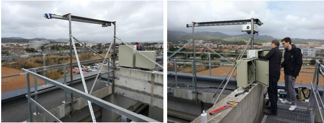
Figure 5.7. The Metallic structure that holds the rail is attached to the building and uses struts to reduce any swing (left). Supplementary electronics are installed in two weatherproof cabinets (right).
