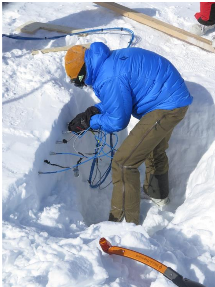
Figure 5 The PT100 probes placed at the same depth for calibration purposes.
