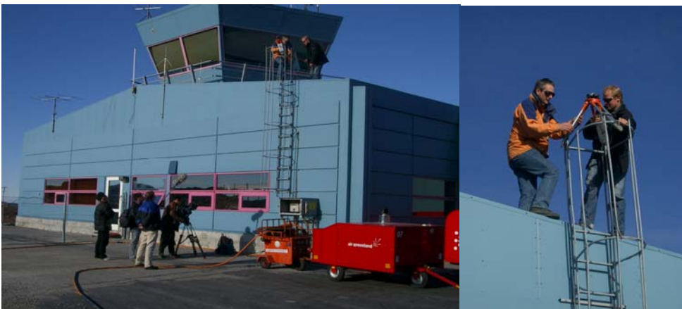
Figure 5.2-3 Ilulissat: DGPS ground station, antenna was installed on top of the fire ladder at the tower. Data was named ILLU.
